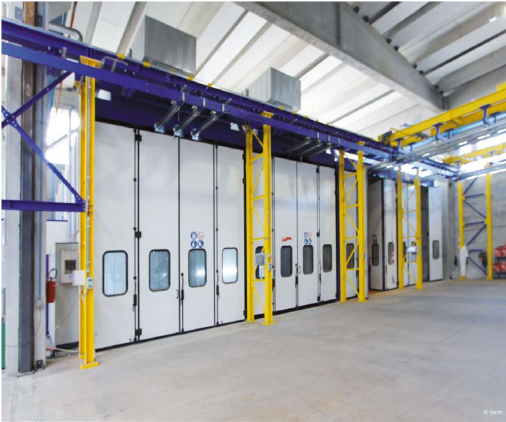
The three curing ovens.
