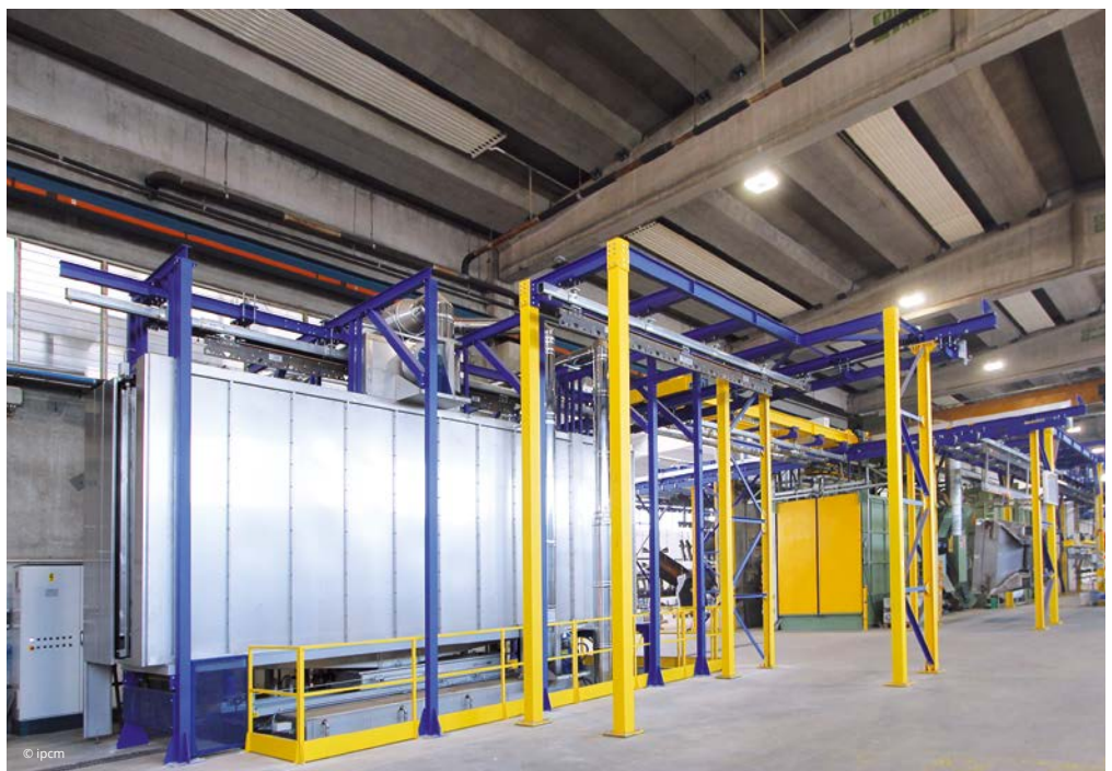
Front view of the Eurotherm coating plant installed at Giletta’s premises. From left to right: the cell cleaning tunnel, the shot blasting machine for large-sized parts, and the loading station.
